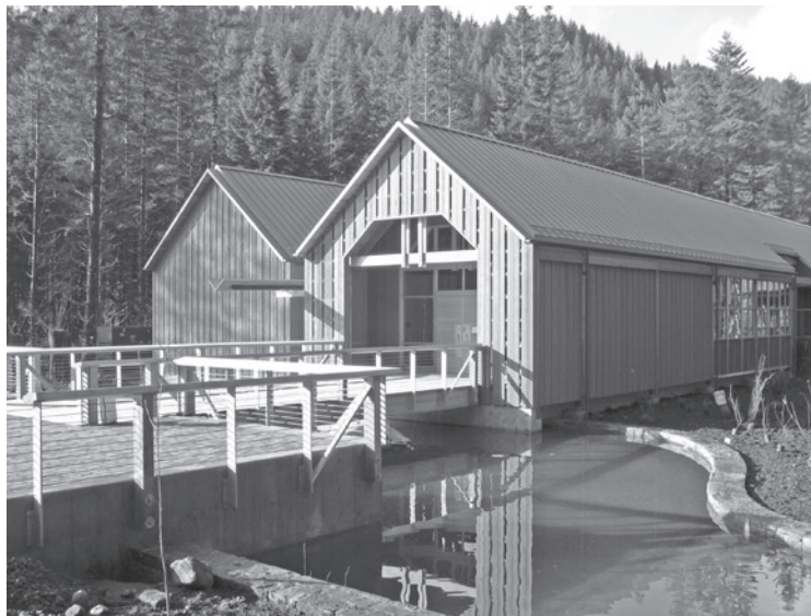
Center construction is nearly complete and exhibit installation begins soon. The view above shows the front entry and fire pond area.
